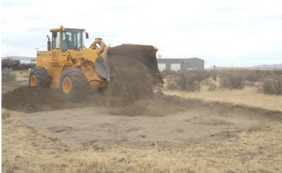
Fig. 3. Filling in the excavations after construction of the site with heavy equipment using the same material that was excavated.
